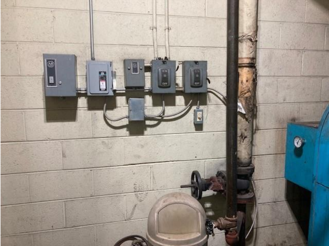
PHOTO 5 – Boiler and Circulator Pumps Electrical and Control Equipment
